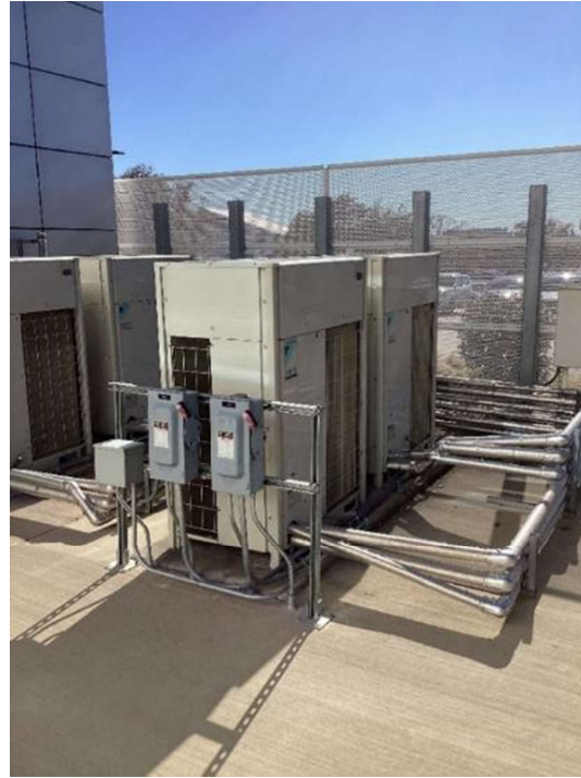
Image 18: Administration Building VRF Condensing Units
