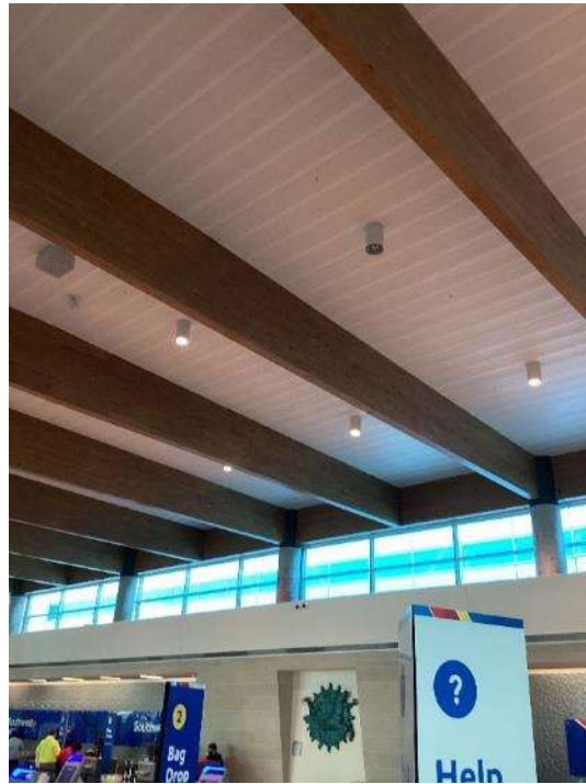
Image 1: Drop Lighting in Terminal Ticketing Area
