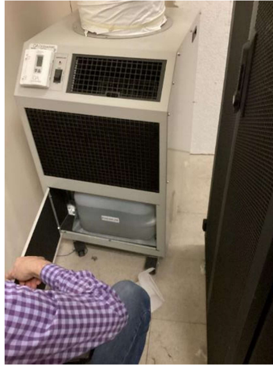
Image 16: Airfield Maintenance Building Data Room De-Humidifier (Full)
