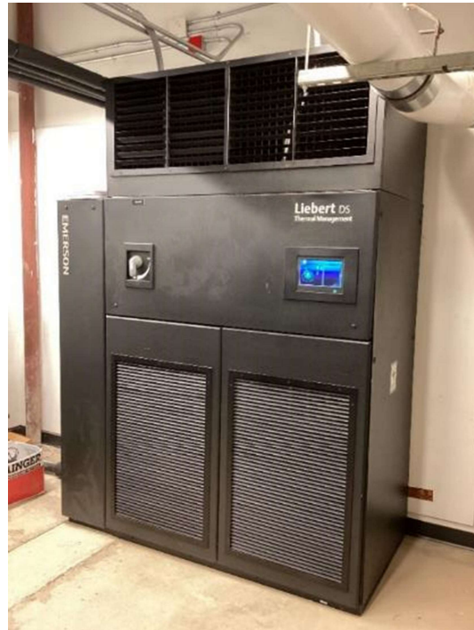
Image 6: Typical Data/Computer Room Unit
