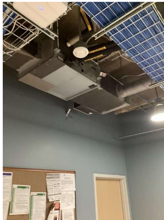
Image 19: Typical VRF Air Handler in Administration Building
