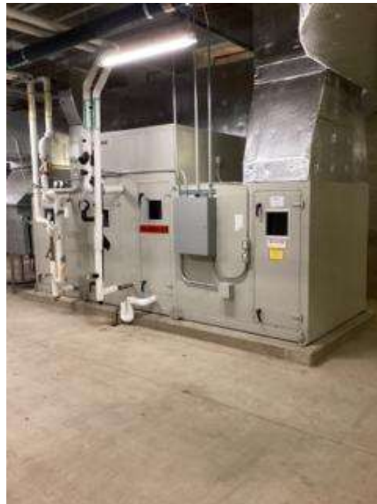
Image 15: Typical Chilled Water/Hot Water Air Handling Unit
