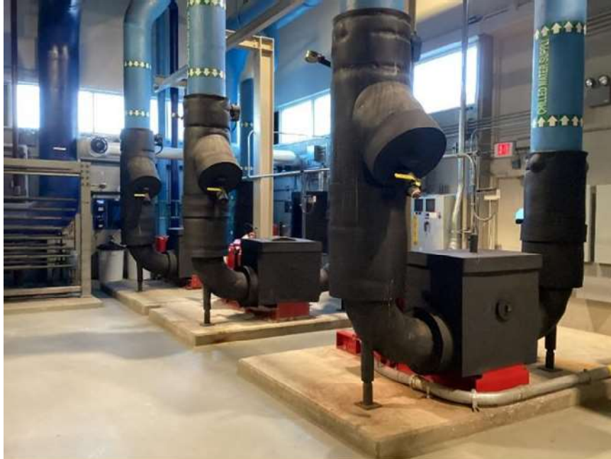
Image 11: Secondary Chilled Water Distribution Pumps (with VFDs)
