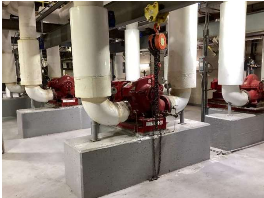
Image 8: Heating Water Pumps
