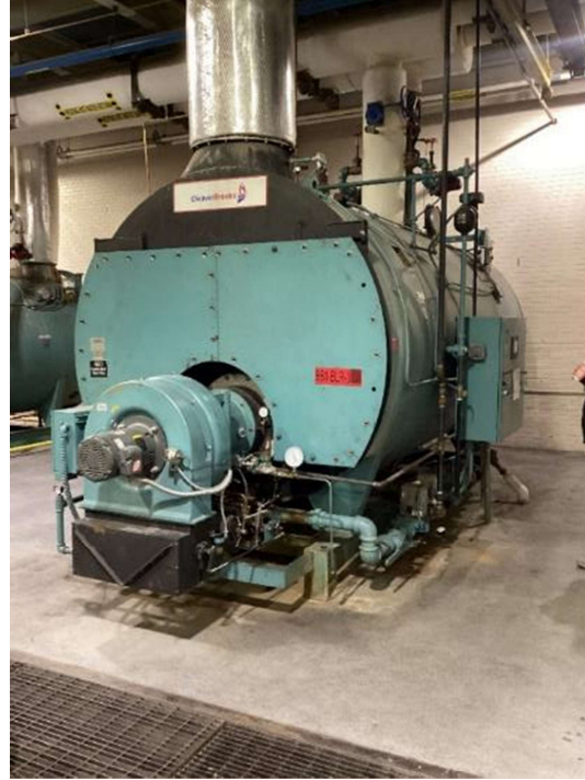
Image 7: Typical Hot Water Boiler
