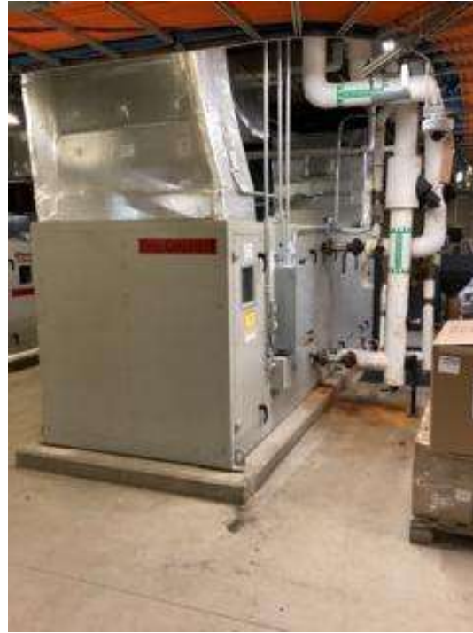
Image 15: Typical Outdoor Air Unit
