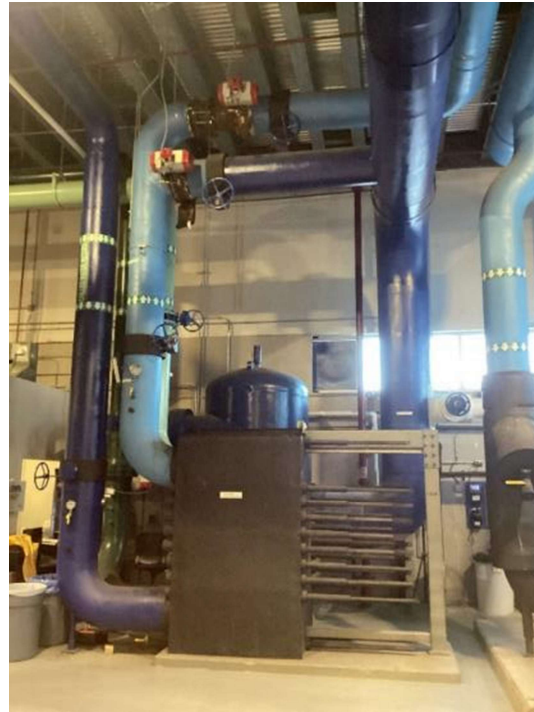
Image 12: Unused Heat Exchanger
